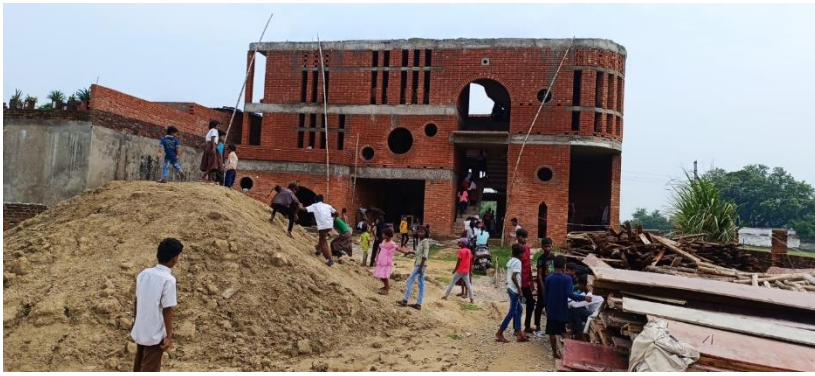
Kids play during recess. They loved climbing the pile of dirt now sitting next to our septic tank.
