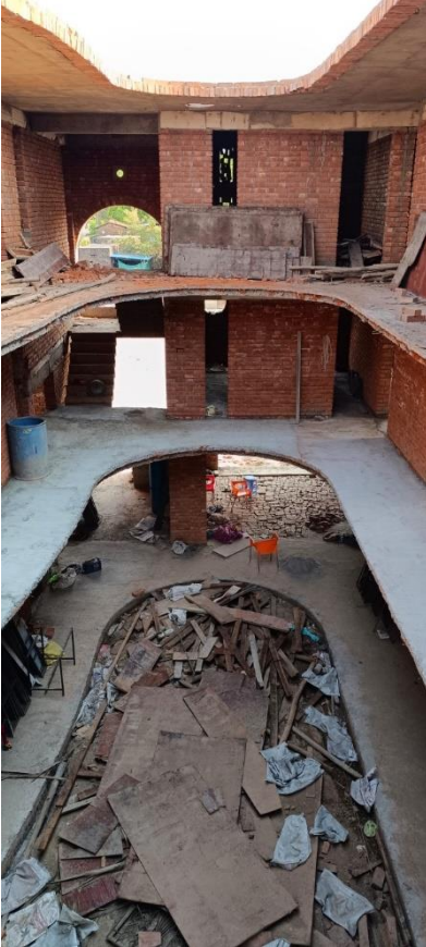
The school one month before opening. Walls complete, but not much else. (this photo taken from back facing front)
