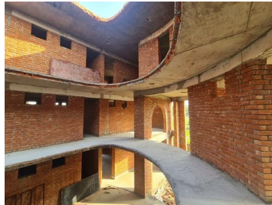
Deep thanks to our architect who designed from the heart. Beautiful shapes and spaces in this building. What a lovely place to grow up! (rear of building)
